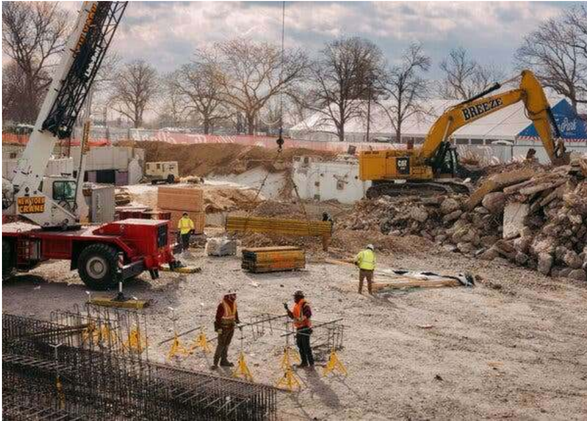
Construction at Belmont Park in Elmont, N.Y., just outside of Queens. Justin Kaneps for The New York Times
